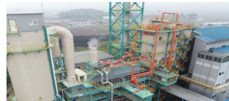
EMKH – Integrated Waste Platform
